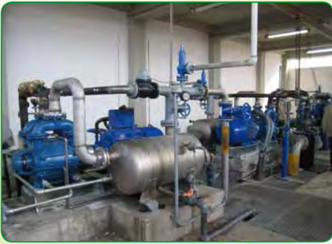
RVS compressor units for BIOGAS circulation in the digester.
